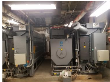
55 Wall Street has 2 BZ Direct Fired Absorption Chillers and a BDH Hot Water Absorption Chiller
